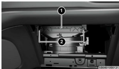
Fresh Air Inlet
